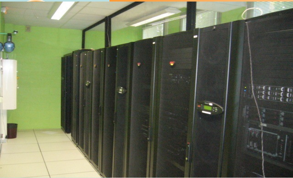
PUE 1.35 Power Usage Effectiveness
